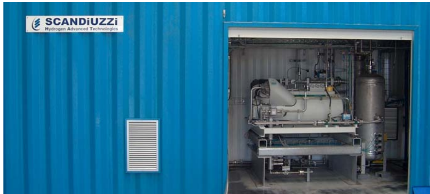
Scandiuzzi hydrogen generator plant with oil-free HAUG compressor
